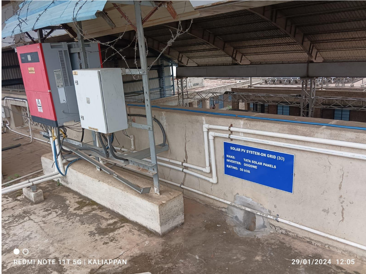
Solar PV System at the top of Main Building
