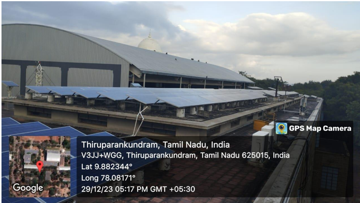
Solar PV System installed at the roof of EEE Department
