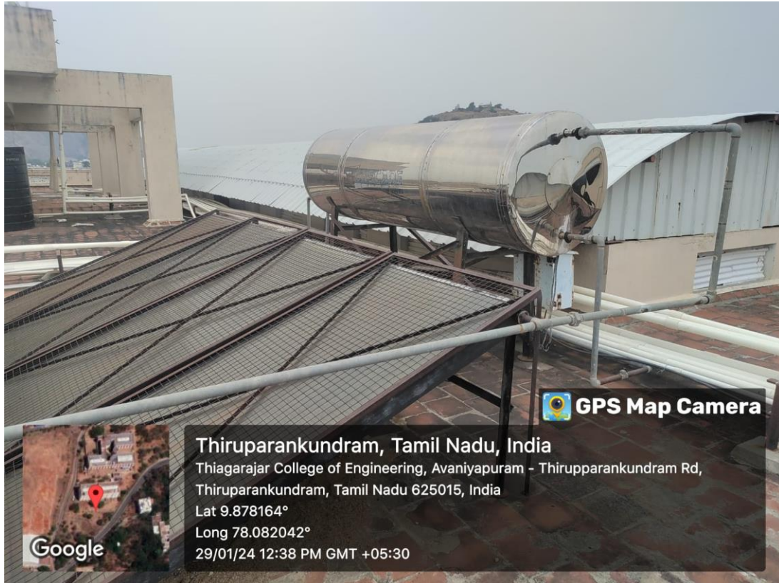
Solar water heater used in the Ladies Hostel Building
